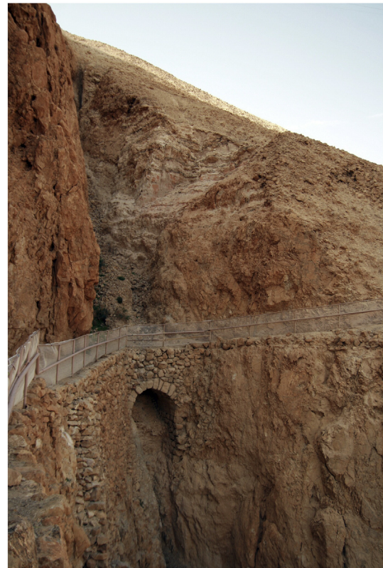
Fig. 13. A general view of the northern segment of the fault bordering the western side of the Masada block and the aqueduct bridge that was built on both sides of the fault. View from the north. Note the good preservation of the bridge, demonstrating the absence of seismic deformation along the fault or in the vicinity of this site since the construction of the bridge during the 1st century BC. Also note the Roman ramp resting on top of the fault with no sign of deformation. The aqueduct bridge, built by king Herold, stretches on both sides of the main western fault of Masada block, ca. 100 years before the construction of the ramp.
