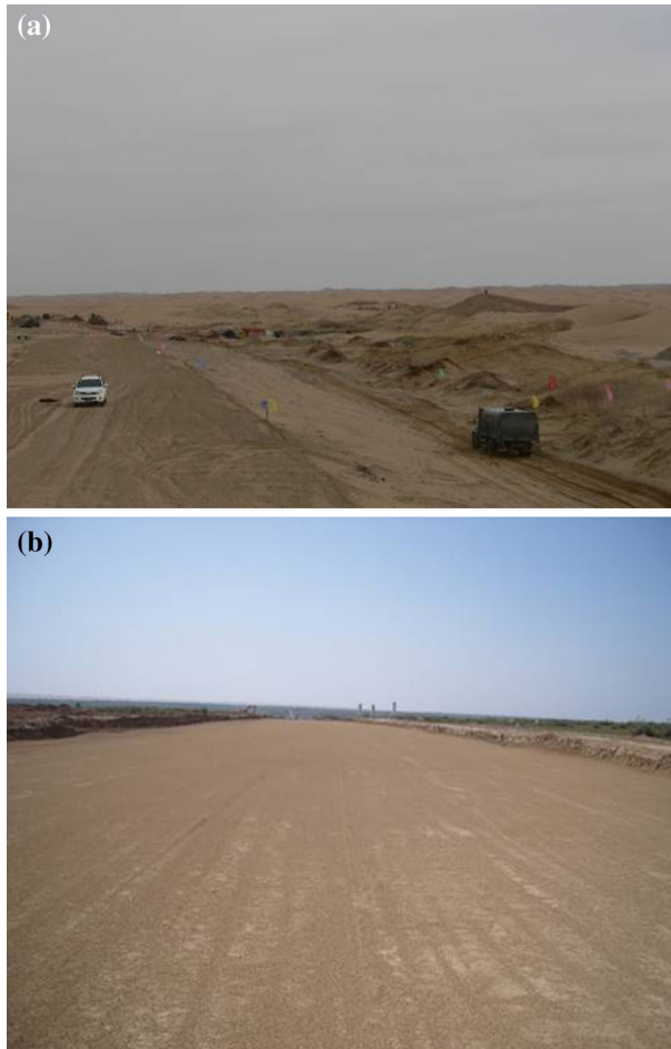
Fig. 2 Yanhuang first-class highway in different construction processes: a before compaction, b after level off and compaction
