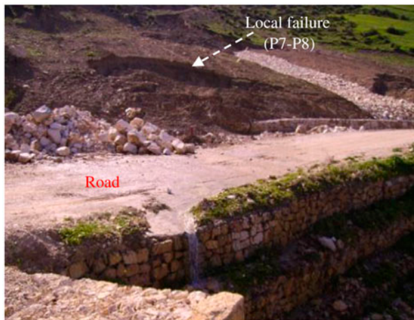
Photo 2. Local failure near the road (this photo was taken at 15 March 2007).
