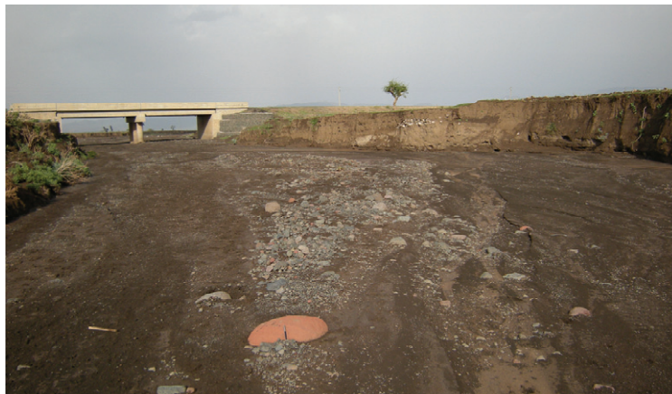
Fig. 3 The measuring site at the Kobo-Alamata road bridge and the river reach upstream. Notice the streambed flat morphology and the scattered large boulders resting on it
